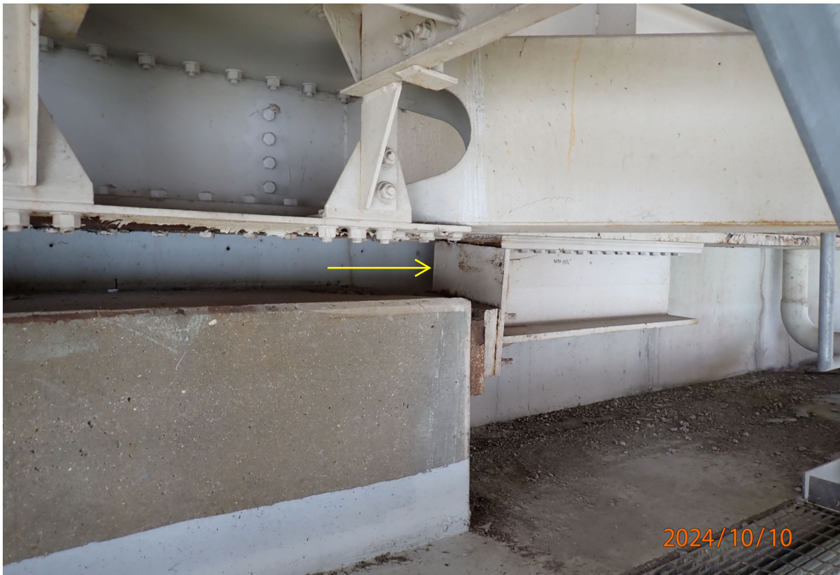
East wind shear beam at Floorbeam 0', Pier 6 (south face) Note bolted plate assembly between wind shear beam and wind anchor concrete is rotated relative to the wind shear beam (see following photo).
