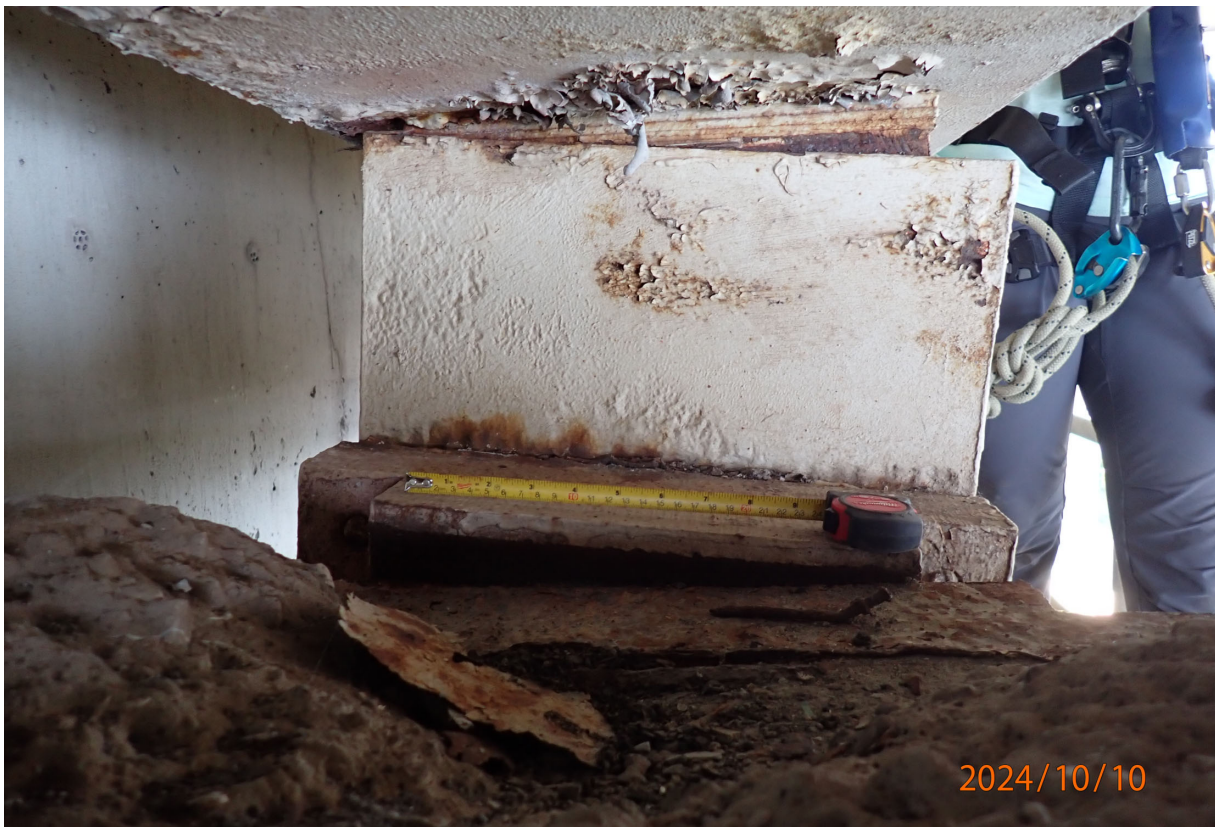
At the west end of the east wind shear beam, the bolted plate assembly is rotated relative to the beam.
