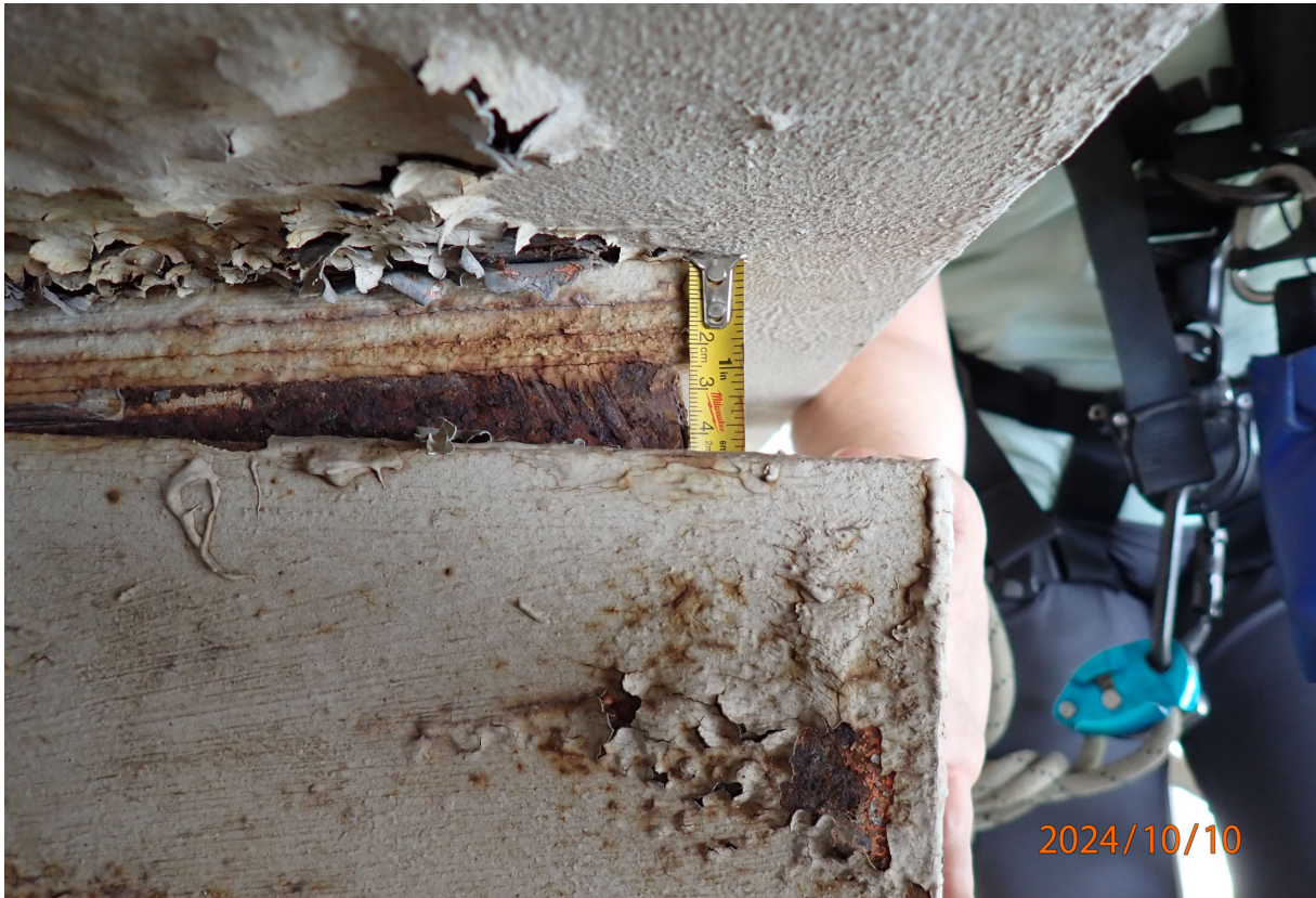
At the west end of the east wind shear beam, the bolted plate assembly is rotated relative to the beam (close up at south side of plate).
