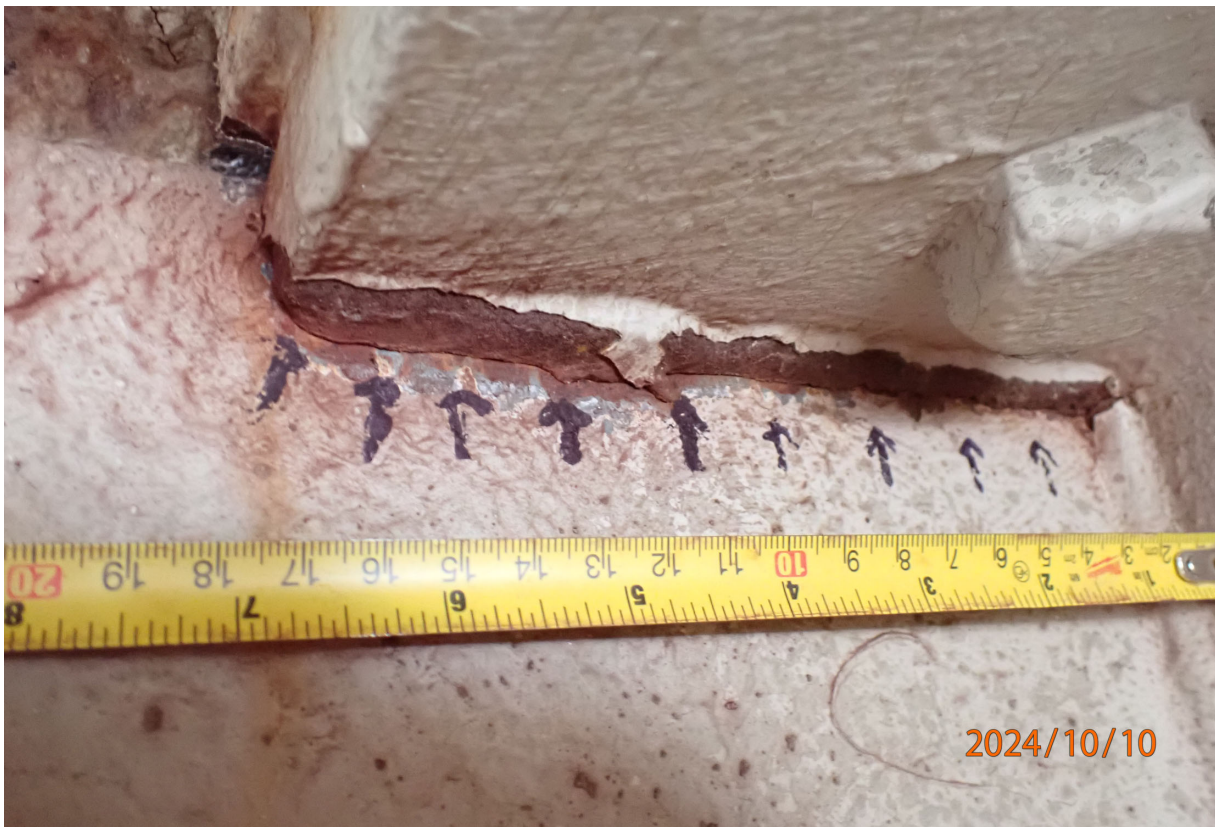
In the west wind shear beam, the north top flange to end plate weld is fully cracked.
