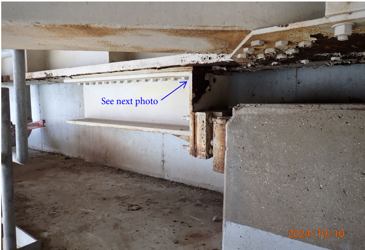
West wind shear beam at Floorbeam 0', Pier 6 (south face) Note bolted plate assembly between wind shear beam and wind anchor concrete is relatively plumb.
