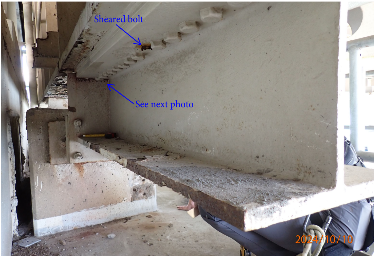
West wind shear beam at Floorbeam 0', Pier 6 (north face) Note sheared bolt in floorbeam bottom flange to wind shear beam top flange connection.
