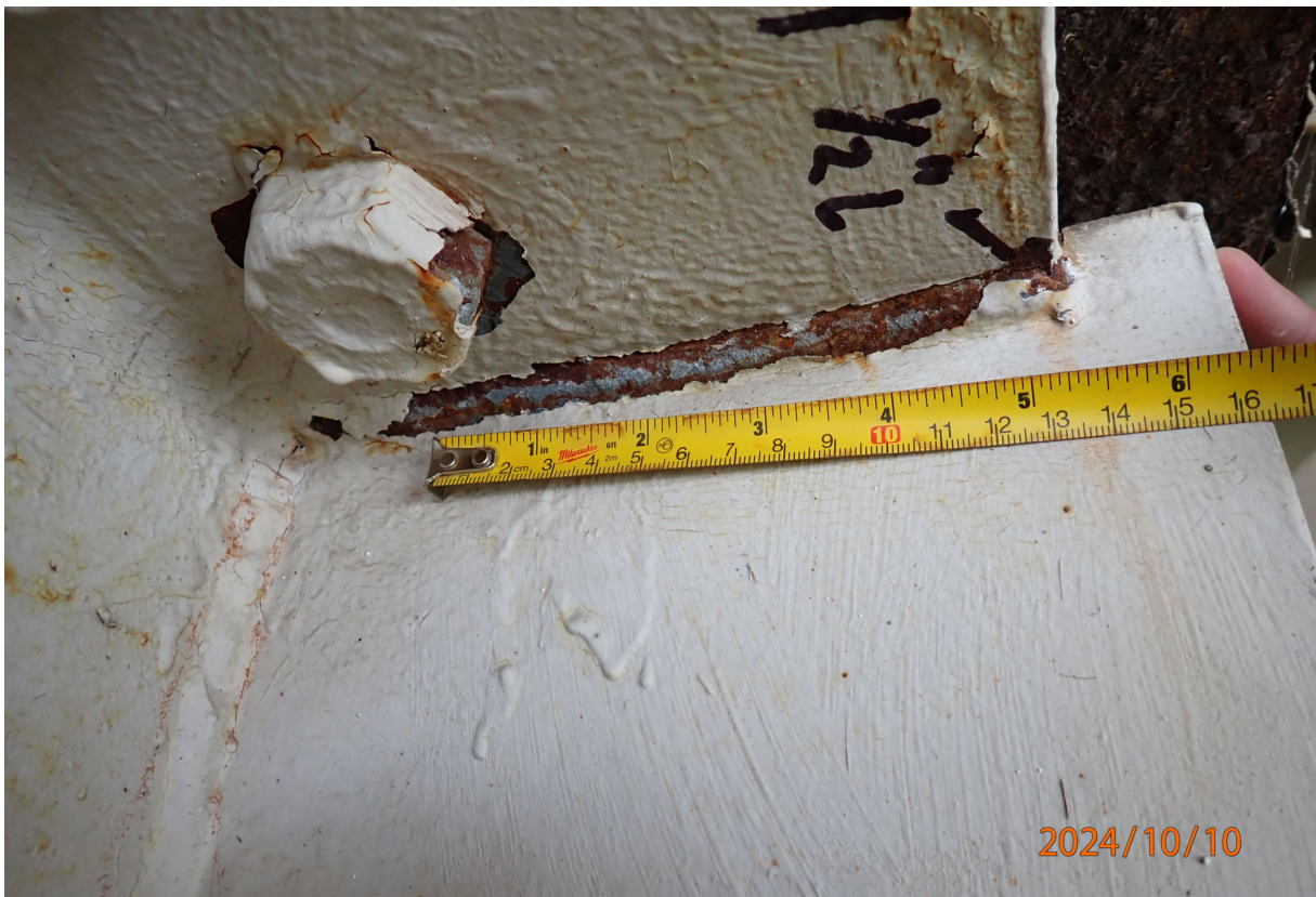
In the west wind shear beam, the top flange to end plate weld has a 1/2" long crack at the south termination (no change).
